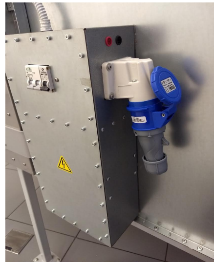
Line filters box
