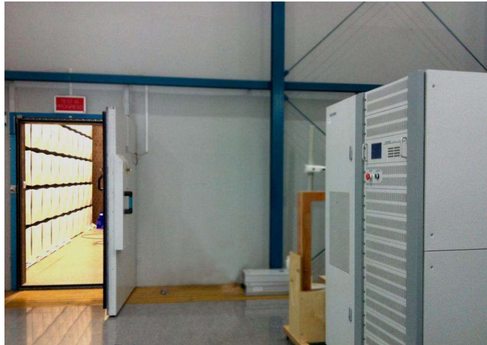
100kVA AC Power Source
